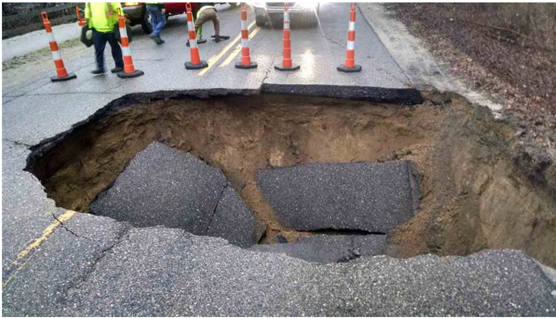
Figure 7. Collapsed section of 148th Avenue in Spring Lake Township after a culvert failure. Image from Grand Haven Tribune online article (link no longer available).
