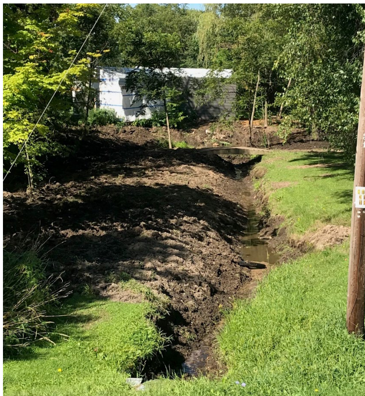
Photo 3. Earth work on the Unnamed Tributary to Huftile Creek downstream of 116th Avenue, Oceana County, August 2020.
