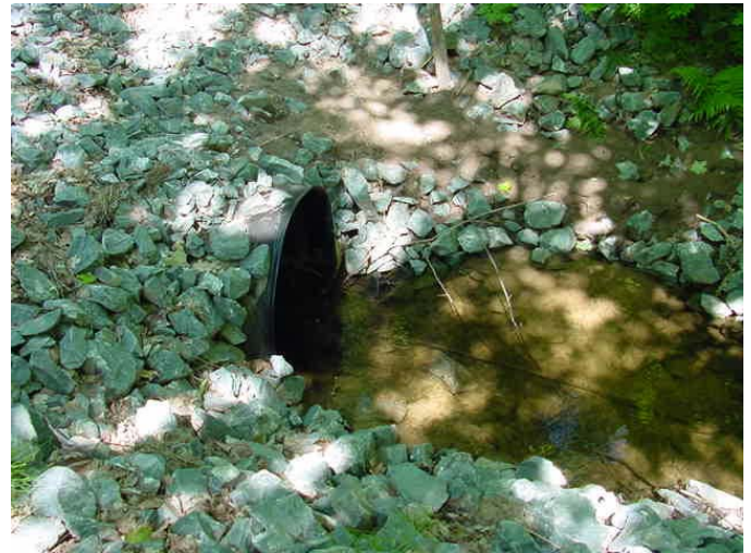
Yellow Dog at Bear Lake Site After: Outlet at Yellow Dog Site, stabilized with 90 cubic yards of riprap.
