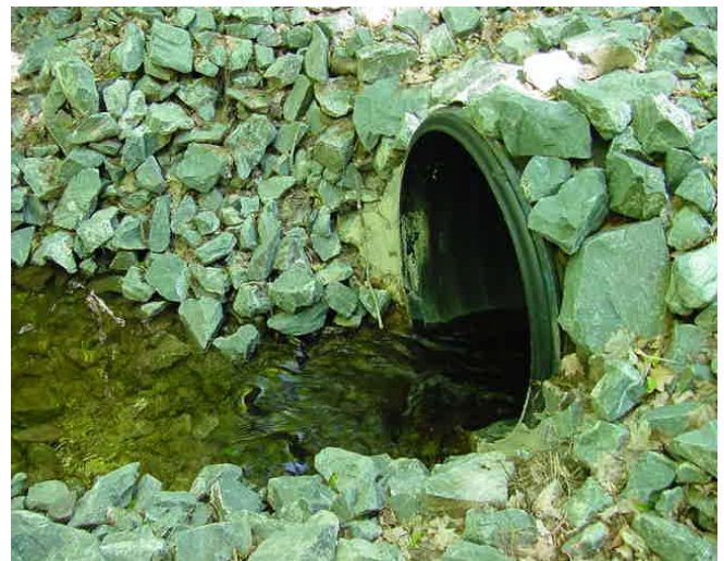
Yellow Dog at Bear Lake Site After: Yellow Dog site stabilized with 90 cubic yards of riprap along with 100 cubic yards of soil and vegetation.
