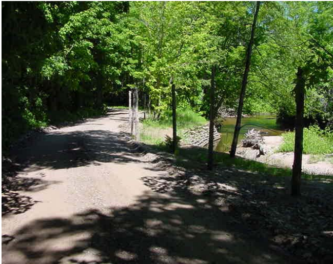
Yellow Dog at Bear Lake Site After: Downstream of the Yellow Dog site stabilized with 130 foot rock crib wall.
