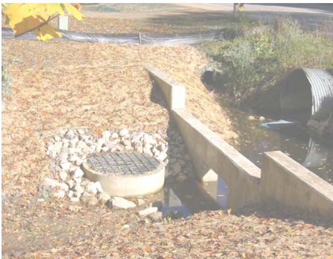
Description: A Diversion structure, where water is channeled into the culvert, which discharges into an infiltration basin, at right.
