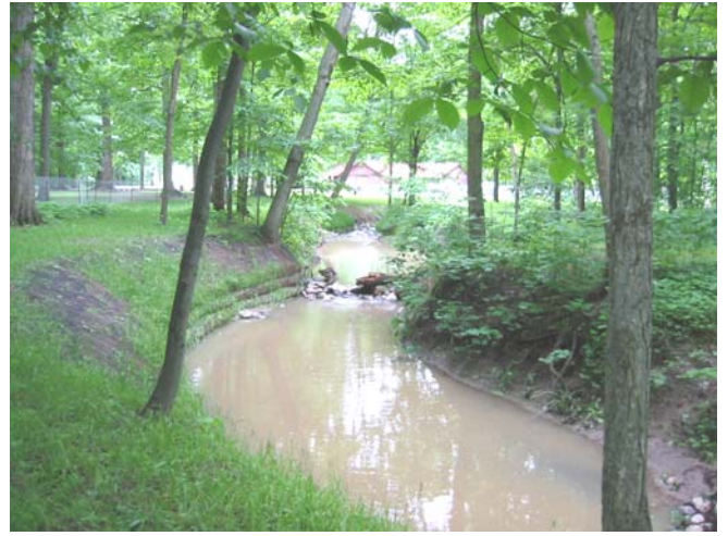
After: Hager Creek Channel banks are restored with geogrid and vegetation and the channel is redirected with the riffle.
