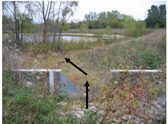
Above: This detention basin holds and treats storm water from traditionally paved parking lot. Right: A rock-lined channel and grade stabilization structure slows down the flow of water and prevents the channel from eroding. Water discharges into an infiltration area.
