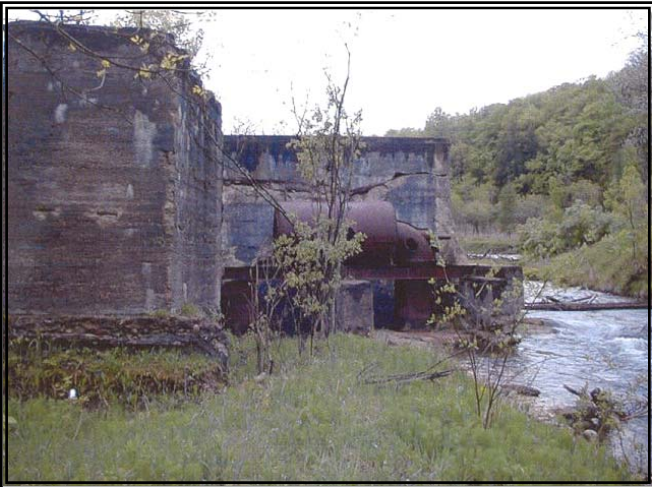
Stover Dam (Cedar River) Before: The remains of Stover Dam after it broke during a series of heavy storms. The failure caused extensive damage downriver
