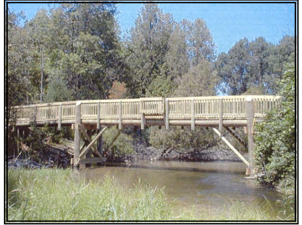
Cedar River "Nature" Bridge After: Here, the old bridge has been removed, allowing for the construction of this new clear span bridge. Rock rip rap and critical area treatment were placed along the river bank.
