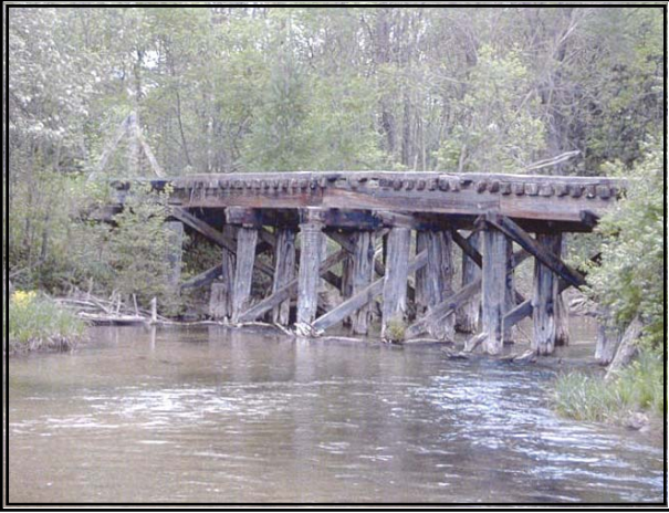
Cedar River "Railroad" Bridge Before: Deteriorated railroad bridge causing erosion and sedimentation.
