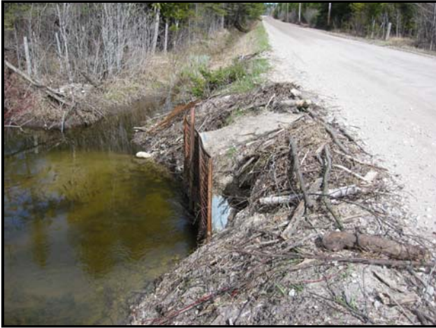
Description: During an inventory of the sources of pollution in the watershed, poorly designed road-stream crossings were identified as a significant source of sediment.
