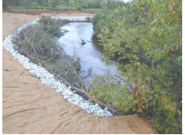
Site 1 after the implementation of an erosion control blanket, rock riprap, and native grass seeding.
