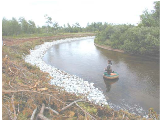
Site 2 after the implementation of 280 feet of lunker structures, brush mattress, riprap, and native grass seeding.
