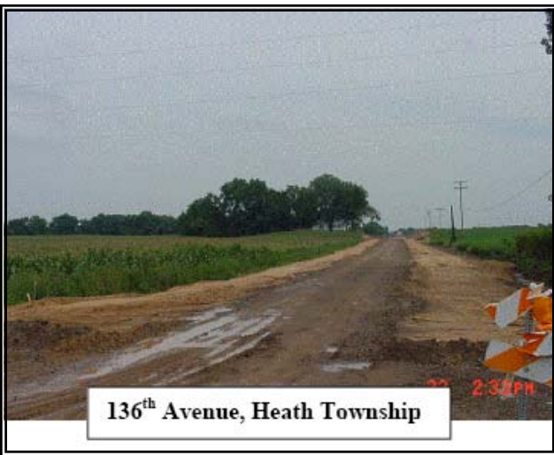
136th Avenue in Heath Township exhibits signs of excessive erosion and was identified in the Watershed Management Plan as a priority site for corrective measures.
