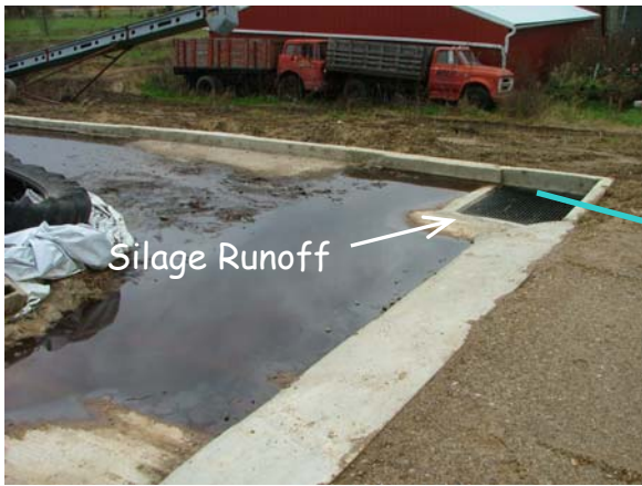
MarGro Farm - after construction, runoff containment prevents groundwater pollution by collecting runoff and discharging it to the waste storage facility.
