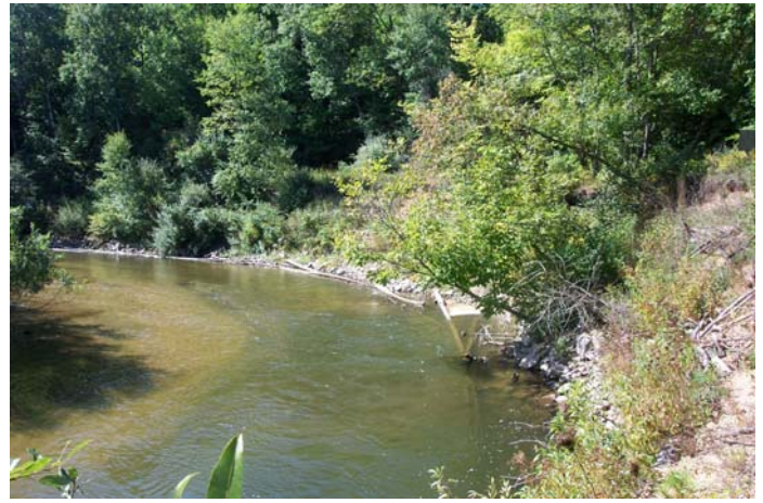
Site #146 After 3 Years: Over 200 cu. yds. of fieldstone were placed along the toe of the bank, log terraces were installed along the upper slope, seedlings were planted, and woody debris was placed in the stream in front of the rock for fish cover.
