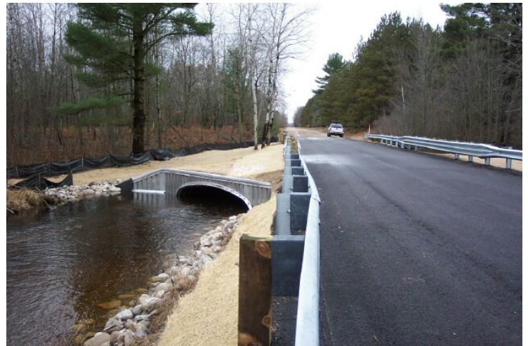
Site #B-17 After: CRA worked with Benzie County Road Commission to replace the 5' diameter culverts with 16' wide bottomless, aluminum arches. The roadbed was paved and diversion outlets installed. Fieldstone and revegetation was incorporated. Now we have a natural stream bottom and the large, unnatural pools at the outlets are filling in and narrowing up.
