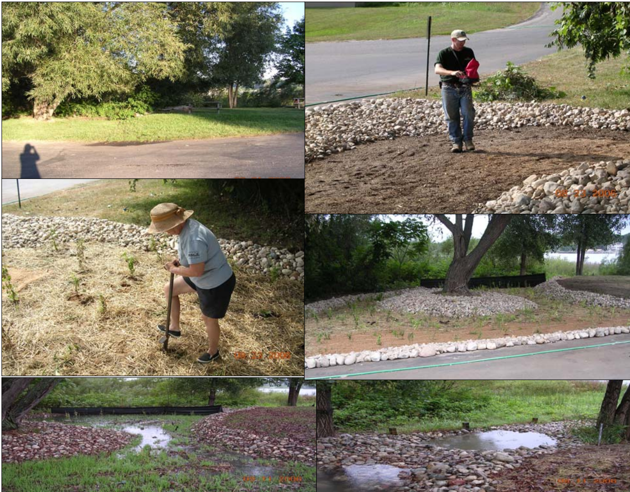
Photo Legend (Mona Lake Boat Club Demonstration Project, August 21-23, 2006): Left to right, top to bottom: Site before excavation work; seeding after rip-rap installation; supplemental plantings; completed project with silt fence upstream of plunge pool; first rain event 3 weeks after project completion; plunge pool holding and slowing water prior to draining into Mona Lake.
