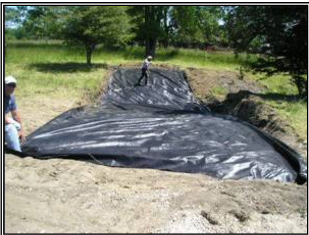
Construction of the livestock crossings involved excavation of the slope to create a gentle grade and the laying of geotextile fabric over which stone could be laid to armor the banks and bottom against cattle hoofs.
