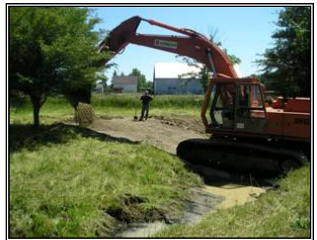
A hydraulic excavator was used to excavate the slopes, apply the stone and even to push in the fence posts. The workmen, who were familiar with cattle, advised that small diameter stone should be used or the cattle might be afraid to walk on it.
