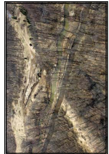
Excavation of the historic channel of the BCR Restoration Project in Charlotte
