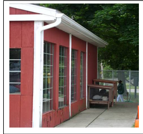
Building with gutters installed. Connected to bioswale.
