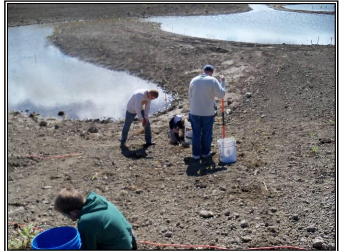
Hollywood Basin During Construction: Volunteers plant native wetland vegetation species at one of three planting days.
