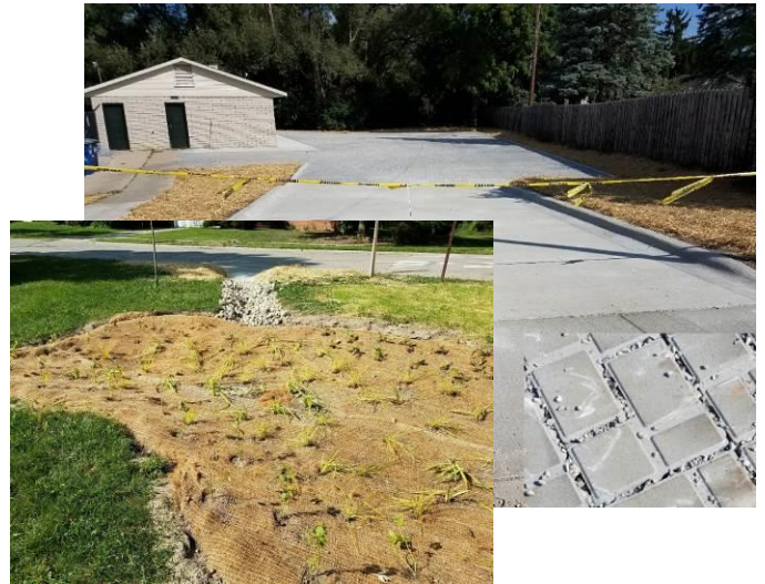
Forestbrooke After: Parking replaced with porous pavers and underground stone basin. 4 bioinfiltration cells receive street and roof runoff.
