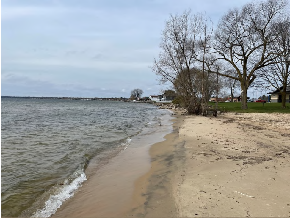
Photo 11: Looking west along the beach toward armored shoreline in HREA C – East Tawas City Park, City of East Tawas.
