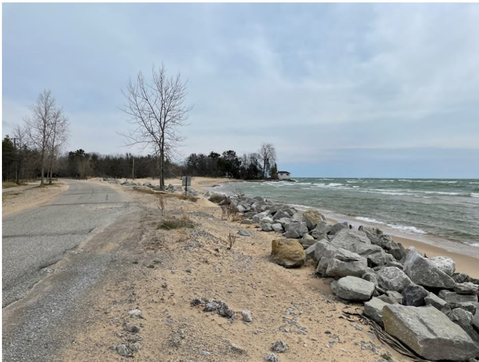
Photo 10: Looking north along EHL in HREA E – Tawas Point State Park, Baldwin Township. Note the recently installed revetment and evidence of erosion damage to road.
