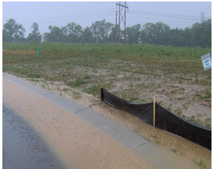
Figure 3 - Sediment discharges from a construction activity.
