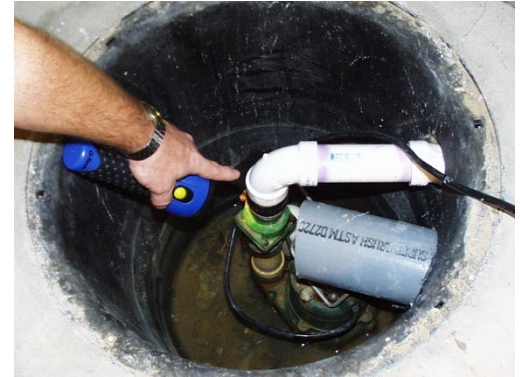
Figure 36 - Ejector pumps in sumps need to be manually operated to prevent unexpected unauthorized discharges.
