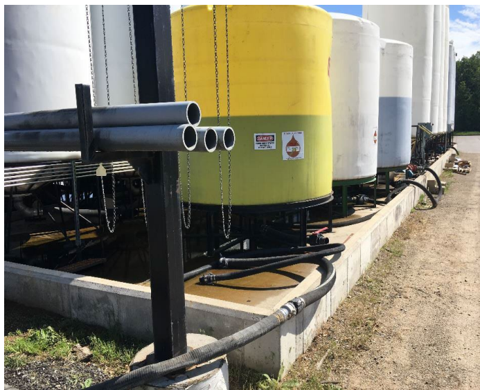
Figure 38 - A STSWCS is required for discharges of storm water to surface waters of the state from regulated secondary containment structures.
