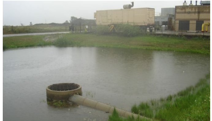
Figure 35 - Detention basins will have an outlet structure that discharges storm water to surface waters of the state.
