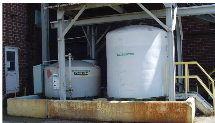
Figure 33 - Secondary containment is intended to protect the environment in the event there is a leak from the storage tanks.
