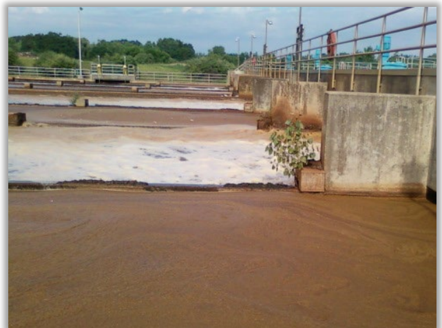
Foam at a treatment plant because of industrial discharge.
