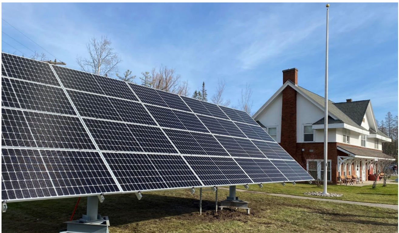
Solar Panels at Oden State Fish Hatchery – photo courtesy of the Michigan DNR
