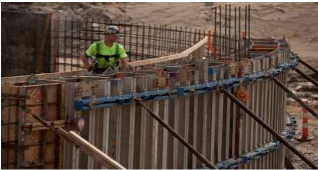
A construction worker works on the wall of a final clarifier at the Ann Arbor Wastewater Treatment Plant on Dixboro Road on Wednesday, Sept. 25.
