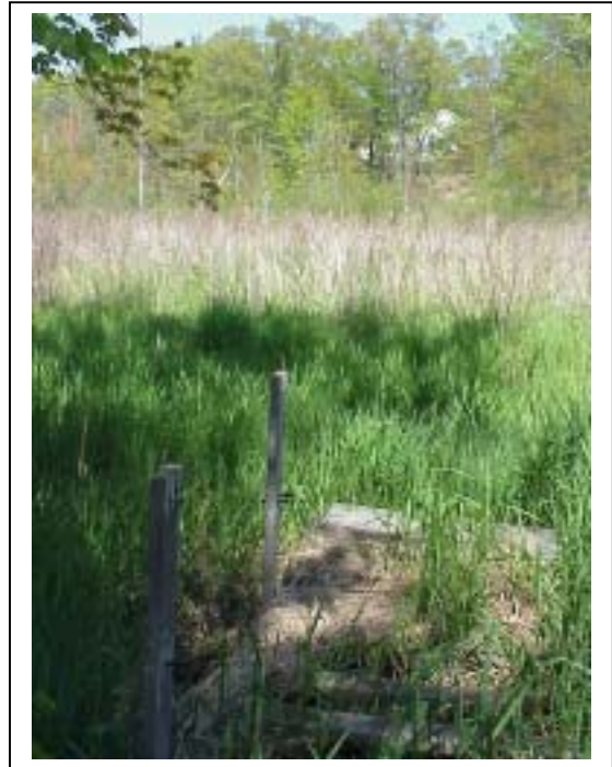
Figure A10. Dilapidated boardwalk overlooking wetland between Johnny O. Harris Park and Mona View Cemetery, Muskegon County, Michigan
