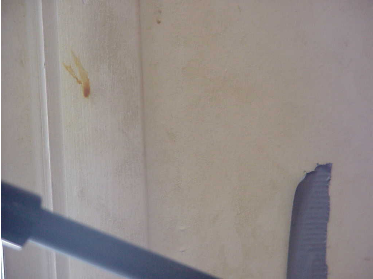
Figure B-4. Visible staining located on the door jamb of the room which was used as the lab. This is likely staining from the iodine solution used as part of the manufacturing process.
