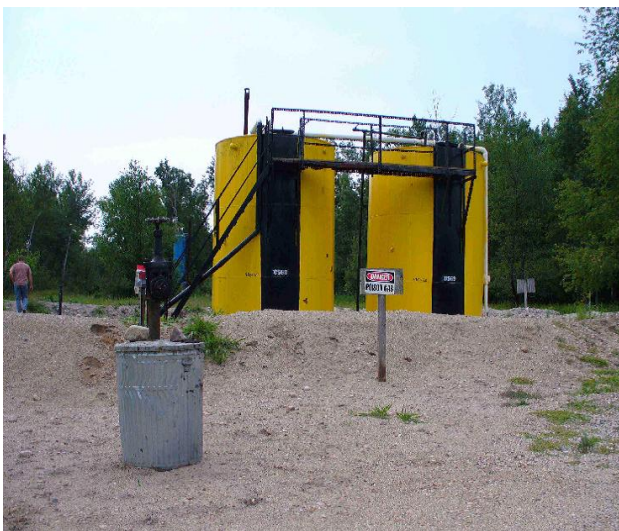
Figure 3: Example of poison gas warning sign around West Branch oil field equipment, Ogemaw County, Michigan.
