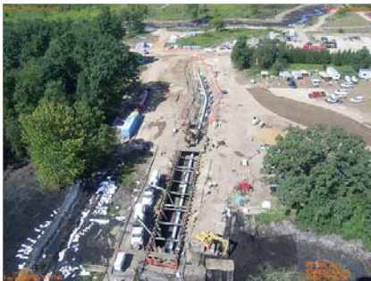
Pipeline break site
