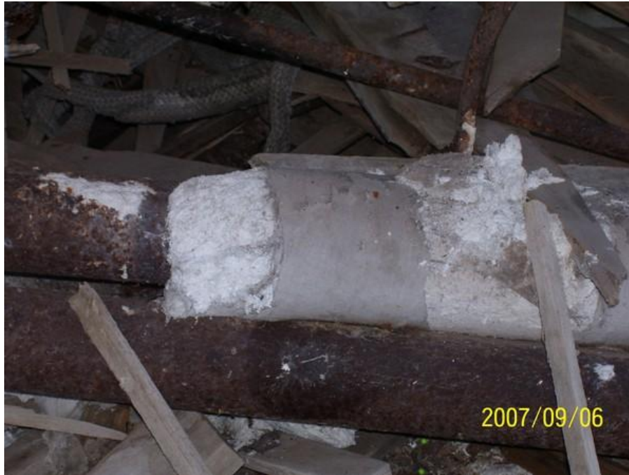
Figure 12. Suspected asbestos-containing material at “Building in Mason,” west of former Quincy Reclamation Plant area (across M-26) in Mason (Houghton County), Michigan. (Picture taken September 6, 2007. Source: Weston2007.)
