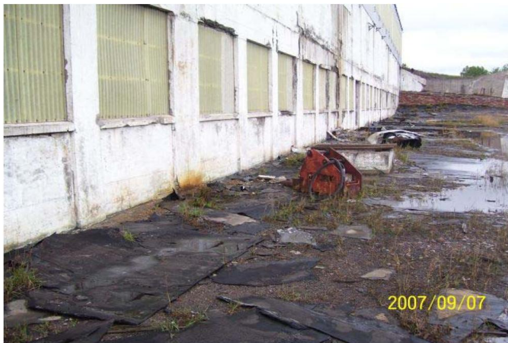
Figure 21. Mineral Building in Hubbell (Houghton County), Michigan. (Picture taken September 7, 2007. Source: Weston 2007.)
