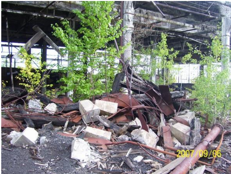
Figure 11. Debris at “Building in Mason,” west of former Quincy Reclamation Plant area (across M-26) in Mason (Houghton County), Michigan. (Picture taken September 6, 2007. Source: Weston 2007.)
