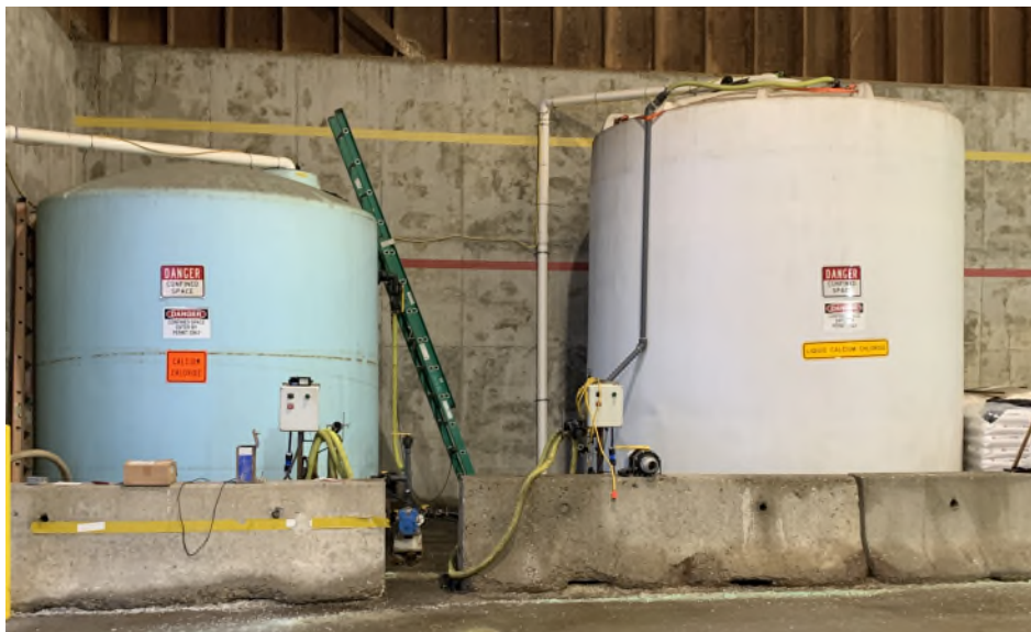
Figure 5.3. Salt Shed Liquid Storage Tanks
