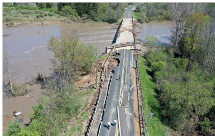
Roadway flooding and damage in Midland County
