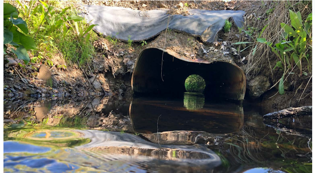
Culvert in poor condition prior to road paving
