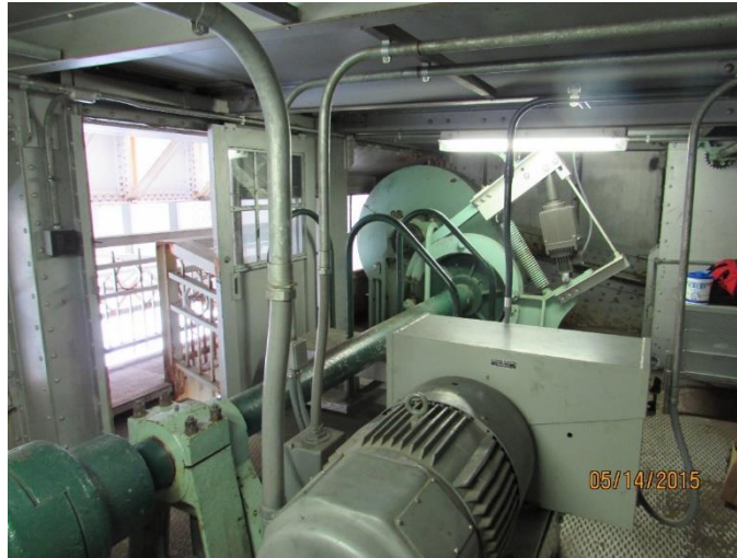
Figure B.03.09 Mechanical System Equipment
