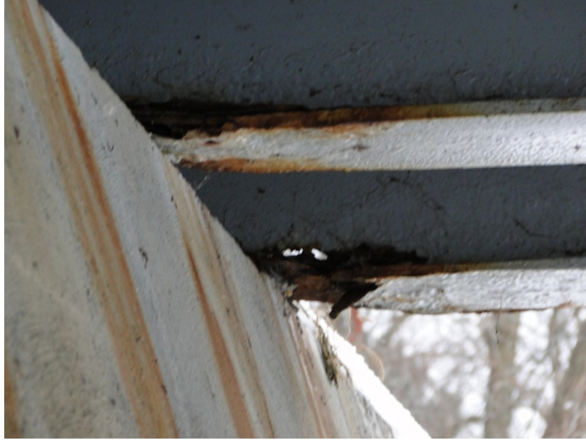
Figure 10.04.01 Severe loss of section resulting in a safe load capacity of 3 tons
