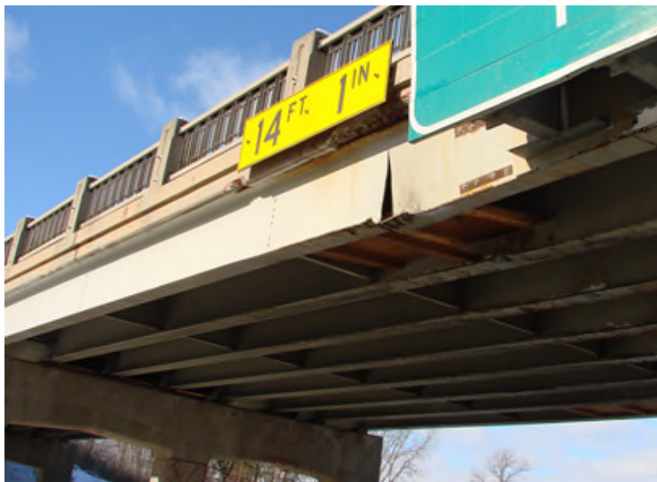
Figure 10.08.01 Crack in fascia beam as a result of a HLH impact
