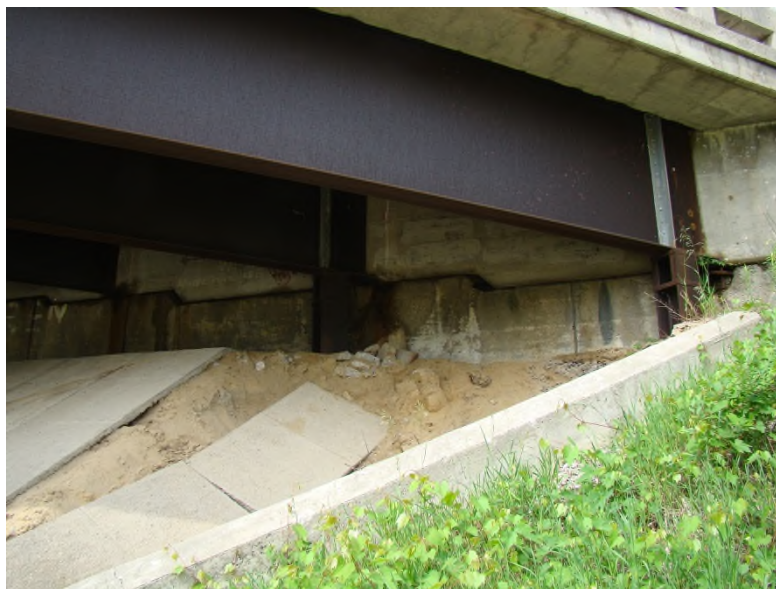
Figure 10.05.01 Load Posting Status should be updated due to temporary supports
