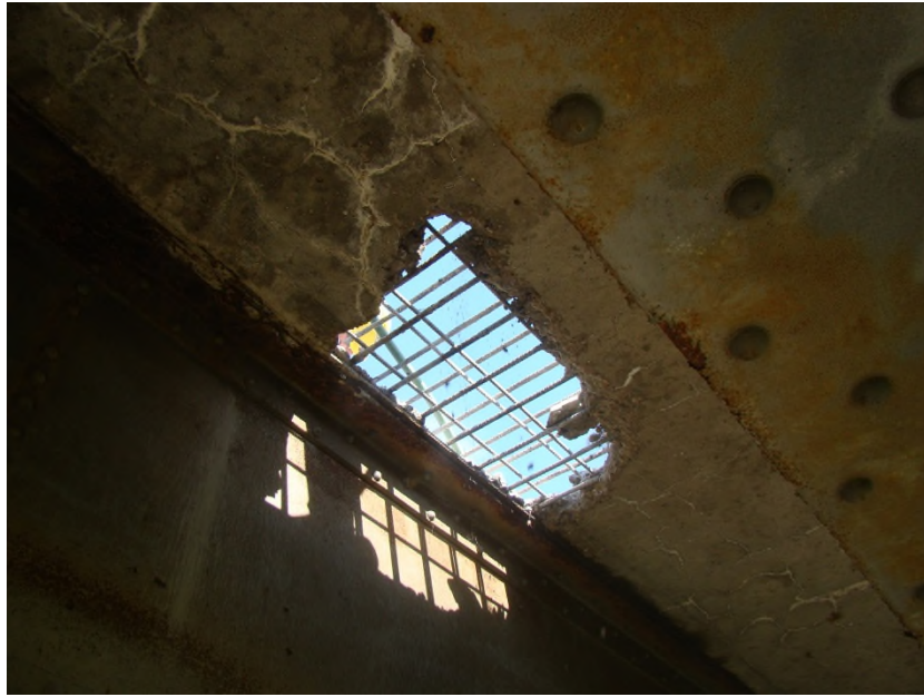
Figure 10.03.01 Full depth hole observed during a routine inspection
