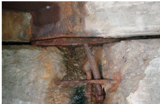
Figure 10.08.03 Abutment spall under fascia beam initiates shoulder closure
