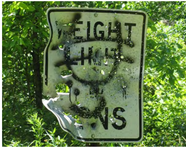
Figure 10.08.02 Bridge posting sign is illegible.
