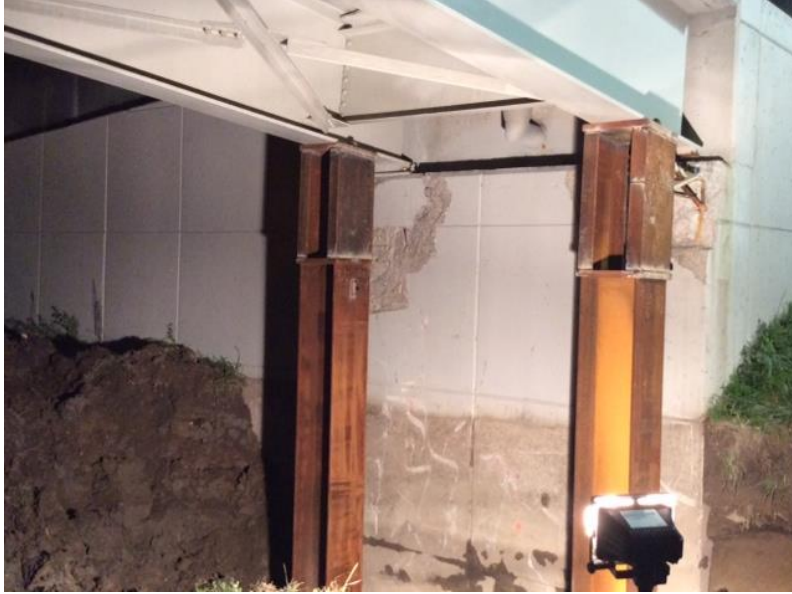
Figure 12.06.01 Loss of Bearing Prompted Immediate Response for Installation of Temporary Supports
