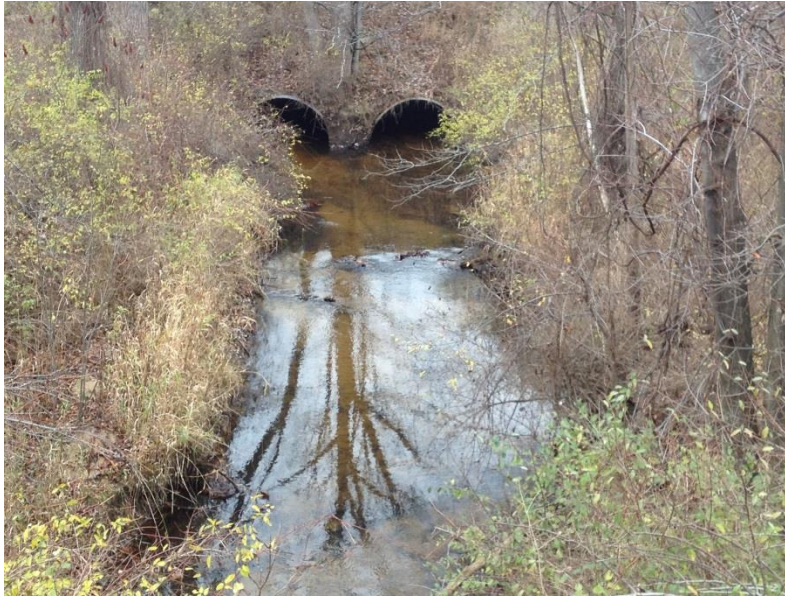
Figure 12.04.01 Double Barrel Metal Culverts that Do Not Meet the Minimum Span Length for the NBI
