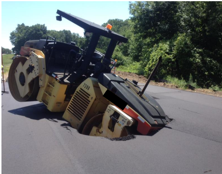
Figure 12.04.02 Failure of Non-NBI Culvert in Poor Condition during HMA Compaction
