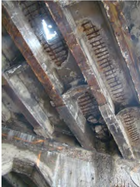
Figure 5.10.02 Deck Bottom Surface in Critical Condition
