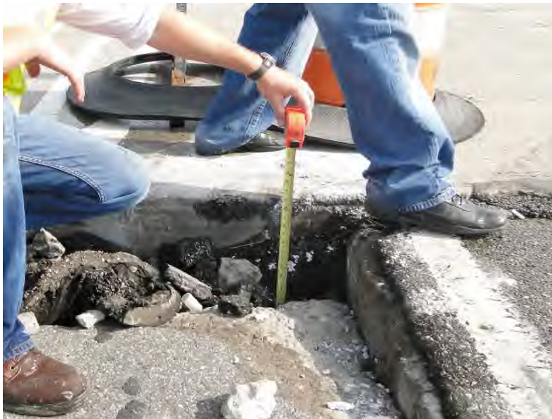
Figure 5.07.03 Failed Approach Slab Resulting from Erosion of Backfill
