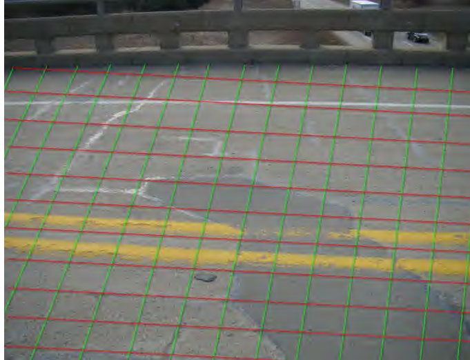
Figure 5.11.02 Element Level Deck Evaluation Consists of Identifying Defects within Each Square Foot of Area
