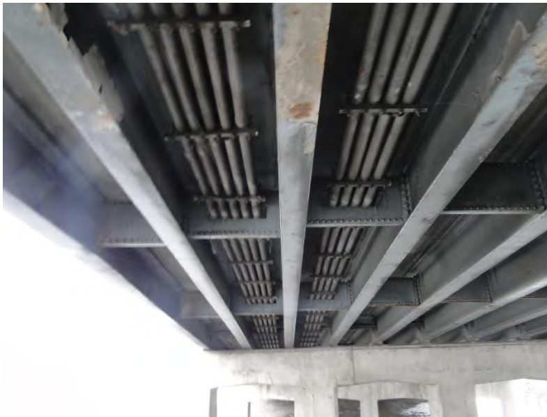
Figure 5.23.01 Telephone Conduit Banks with overhead Adhesive Anchors
