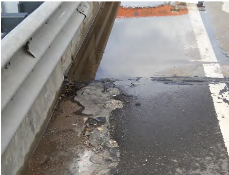
Figure 5.12.01 Ponding Water Near the Reference Line
