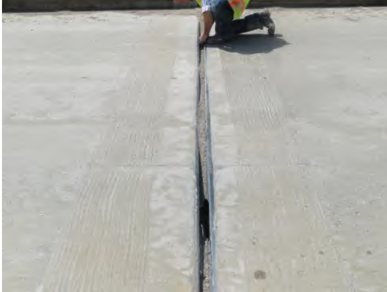
Figure 5.06.12 In-Depth Inspection of Full Depth Strip Seal Gland Failure
