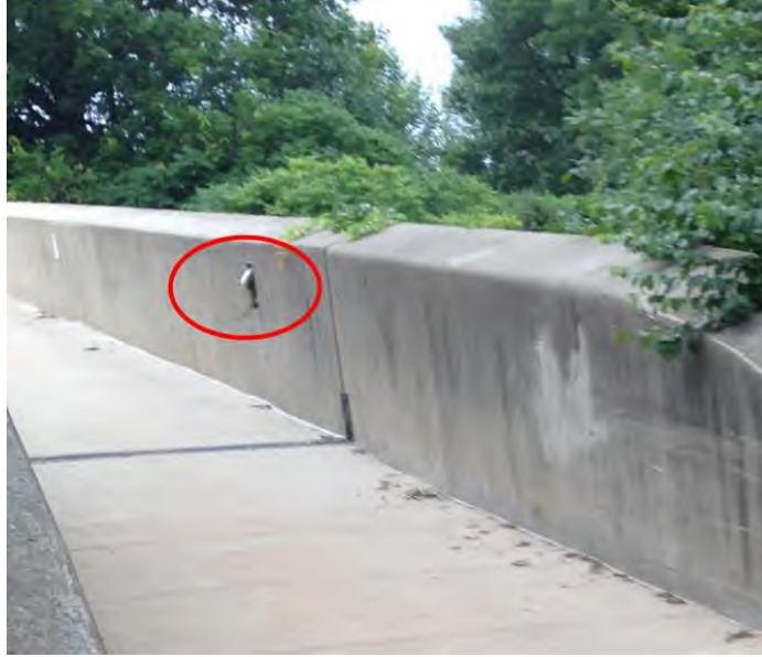
Figure 5.09.06 Damaged Steel Electrical Junction Box Cover May Injure Pedestrians
