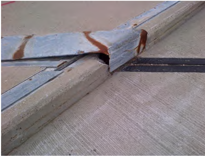
Figure 5.09.01 Damaged Steel Sliding Plates Present a Hazard for Pedestrians
