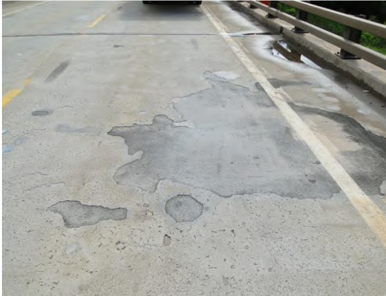
Figure 5.11.01 Deteriorated Thin Overlay with No Defects Observed in the Structural Deck
