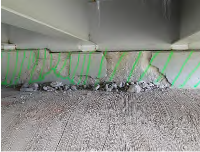
Figure 5.17.06 Severe Abutment Spalling Caused by Pavement Pressure
