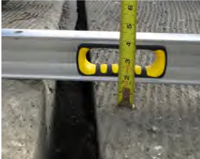
Figure 5.20.01 Approach Slab Settlement at Pavement Seat
