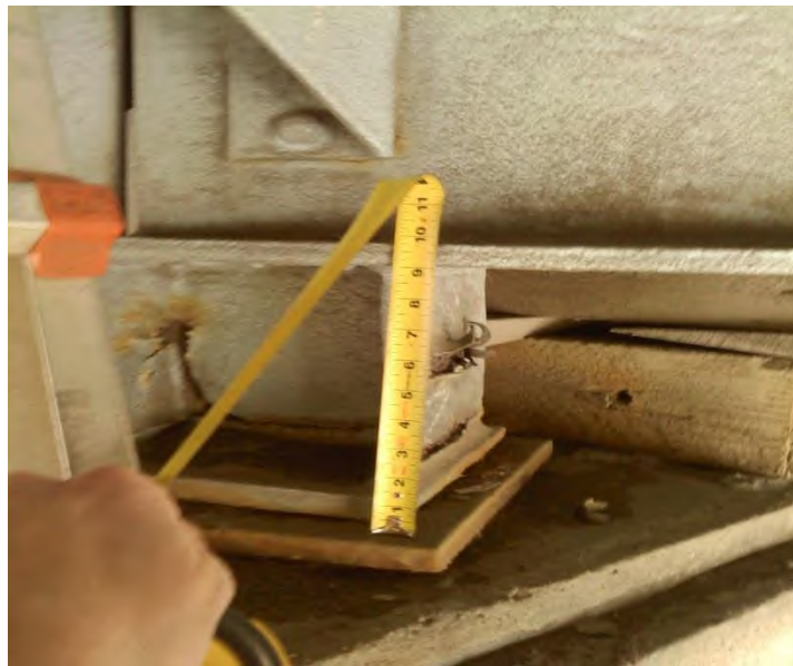
Figure 5.16.08 Cracked H-Bearing Necessitates Detailed Inspection
