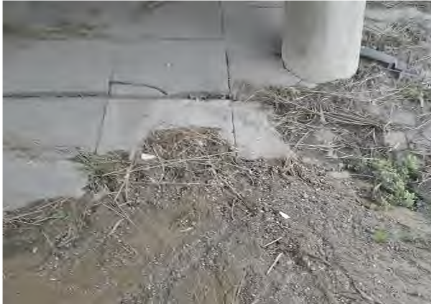
Figure 5.19.01 Loss of Approach Roadway Embankment Fill
