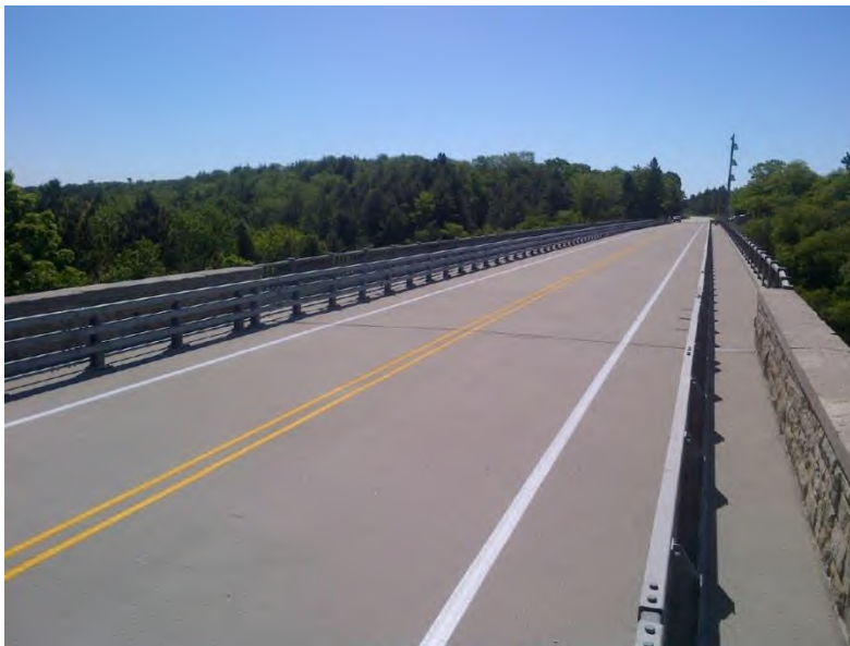
Figure 5.05.02 Thin Overlay Applied to Preserve the Surface of Cut River Deck Truss
