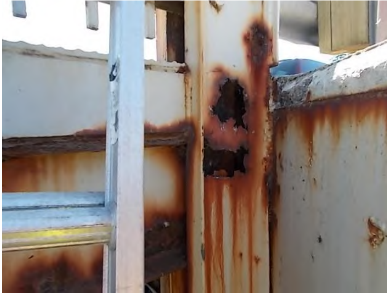
Figure 5.08.26 Steel Railing Posts in Condition State 4 Require Documented Review
