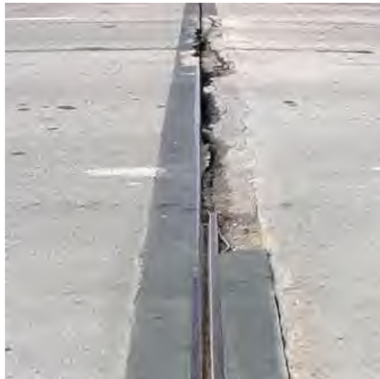
Figure 5.06.11 Failed Expansion Joint and Surrounding Concrete Deck Necessitating Repairs Prior to the Next Schedule Inspection
