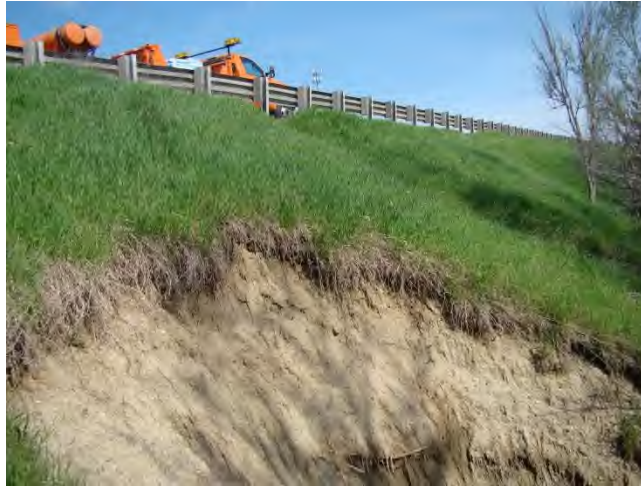
Figure 5.22.01 Washout Discovered Near Approach While Performing Deck Patching
