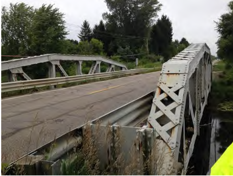
Figure 5.05.04 HMA Wearing Surface applied to the concrete deck of a Pony Truss Programmed for Replacement
