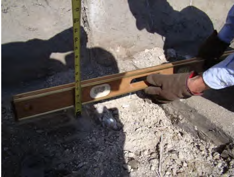
Figure 5.25.01 Settled Approach Basin Full of Debris
