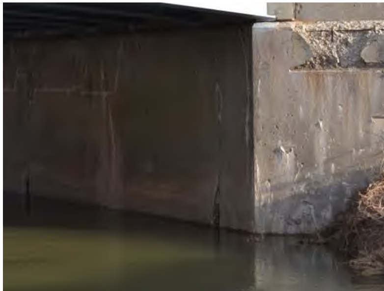
Figure 5.17.01 Abutment with Monolithic Wingwall Deterioration included with Rating of Abutment
