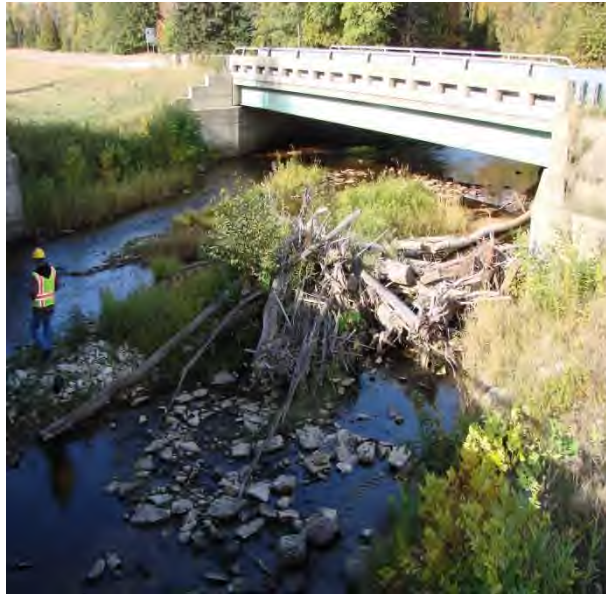
Figure 5.24.01 Debris Accumulation Should Be Included in the Channel Rating
