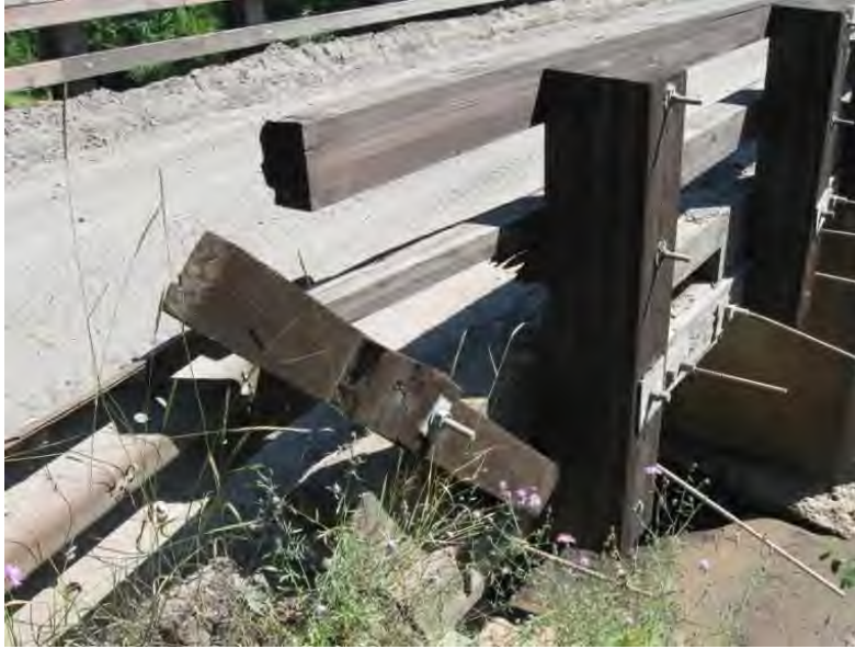
Figure 5.08.25 Timber Railing Damage at the Transition Connection
