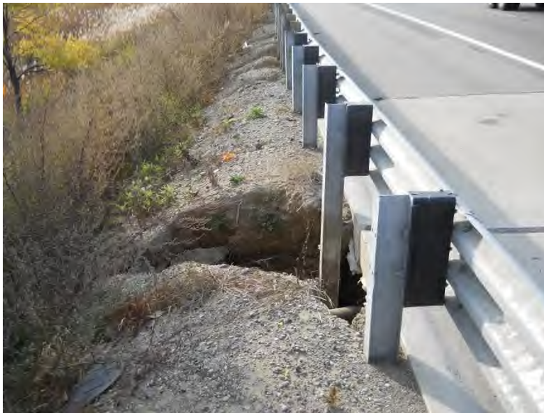
Figure 5.07.02 Erosion Induced By Missing Pressure Relief Joint Material
