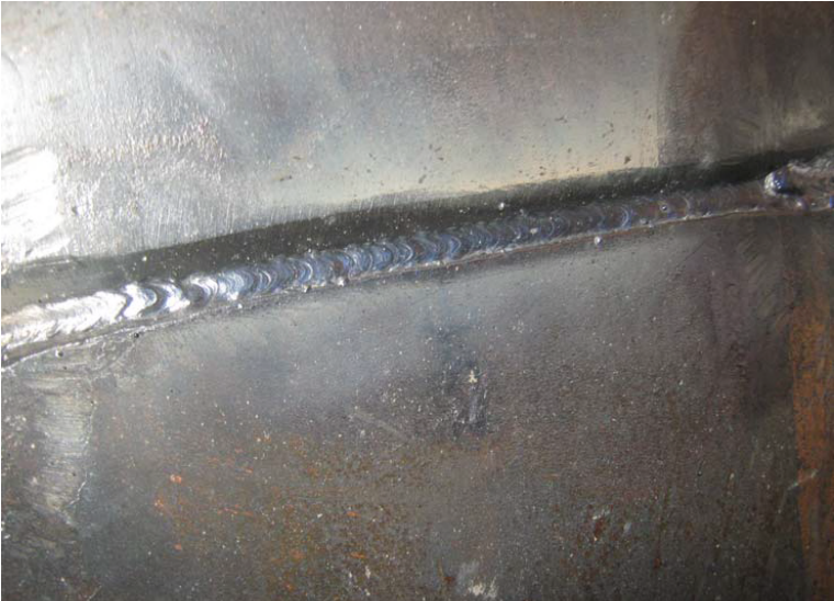
Figure 27. Root pass of a full penetration groove weld free of slag and ready for additional passes.
