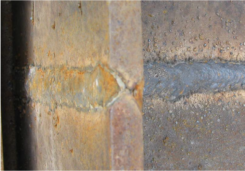
Figure 33. Insufficient back gouging and incomplete penetration.
