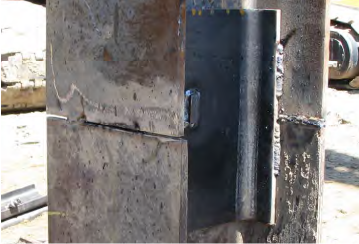
Figure 31. Improper root opening, unprepped surfaces, pile misalignment.
