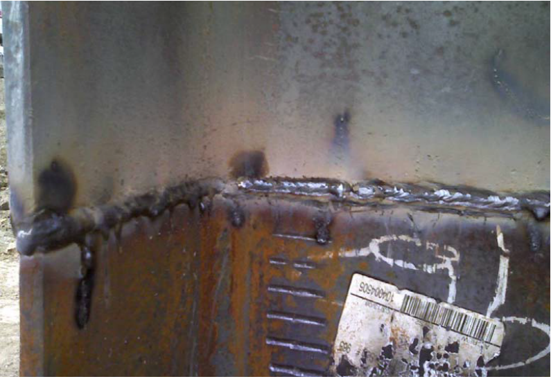
Figure 37. Slag, undercut, underfill, and arc strikes.
