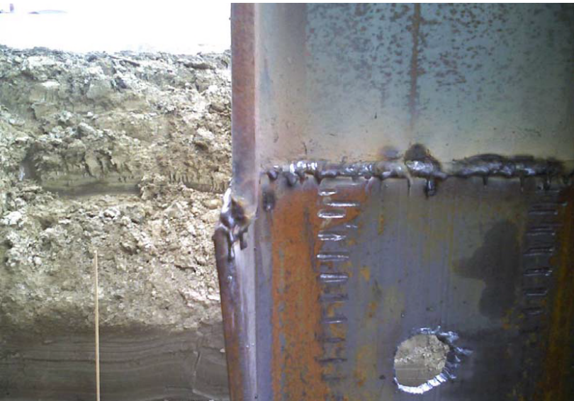
Figure 36. Misalignment, unacceptable profile, slag.
