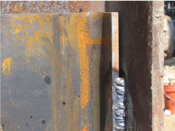
Figure 32. Excessive gap between splicer and pile, incorrect location of fillet welds.
