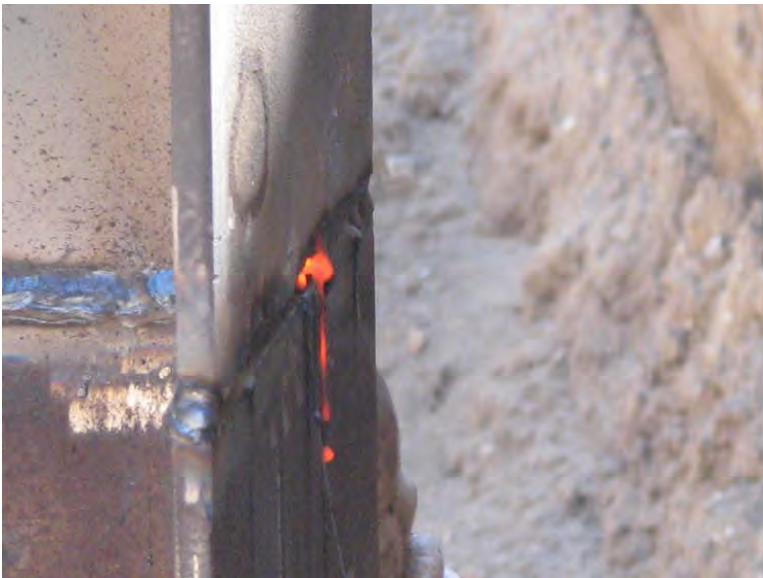
Figure 26. Welding in process. Note slag to be removed to sound metal by back gouging.
