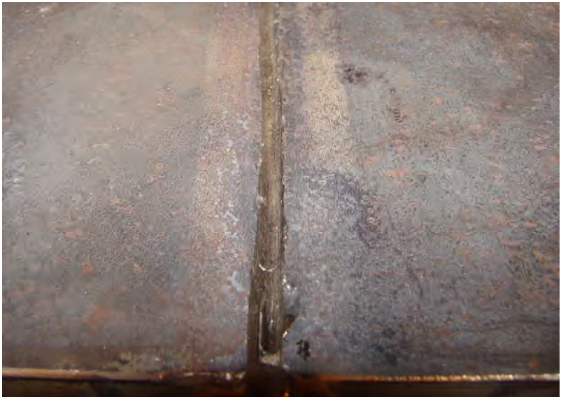
Figure 24. Back gouged to sound metal.
