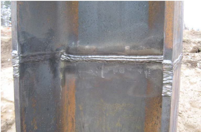
Figure 30. Completed full penetration groove weld. Note that all slag and arc strikes have been removed. Grinding and additional weld metal was added on the flange edges to correct minor misalignment.
