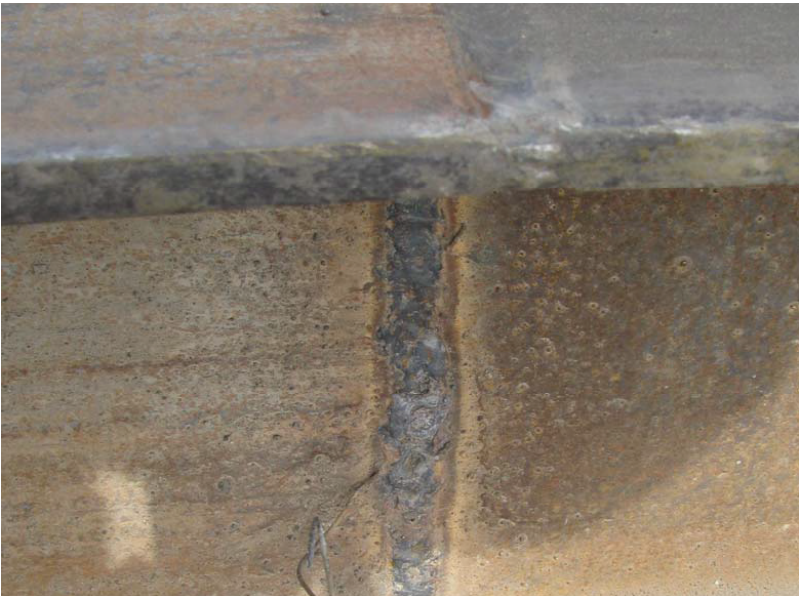
Figure 38. Underfill and use of an unapproved wire fed process (GMAW). Note wire protruding from weld.
