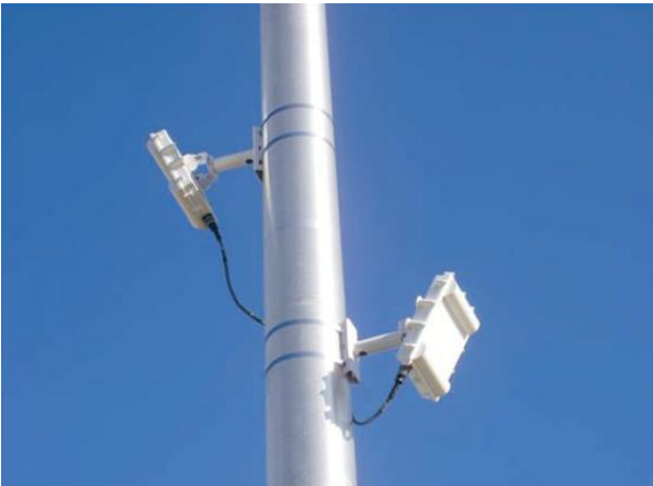
Figure 10 - MVDS Sensor Shown on Roadside Pole
