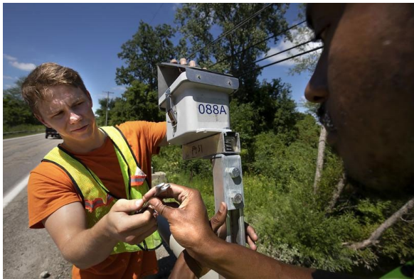
Figure 7. Mitchell Wojtowicz and Kenneth Ferrell deploying an Open-Storm Sensor
