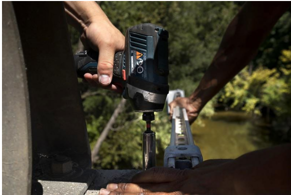
Figure 6. Mitchell Wojtowicz and Kenneth Ferrell deploying an Open-Storm Sensor
