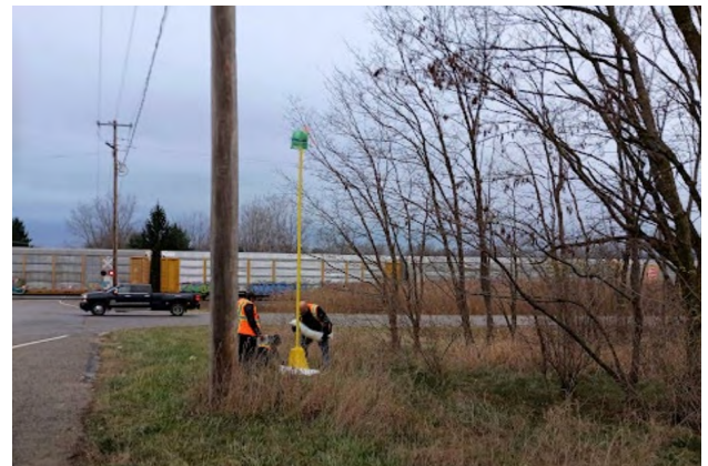
A wireless communications roadside unit is positioned at the southwest corner of the mesh network test area.
