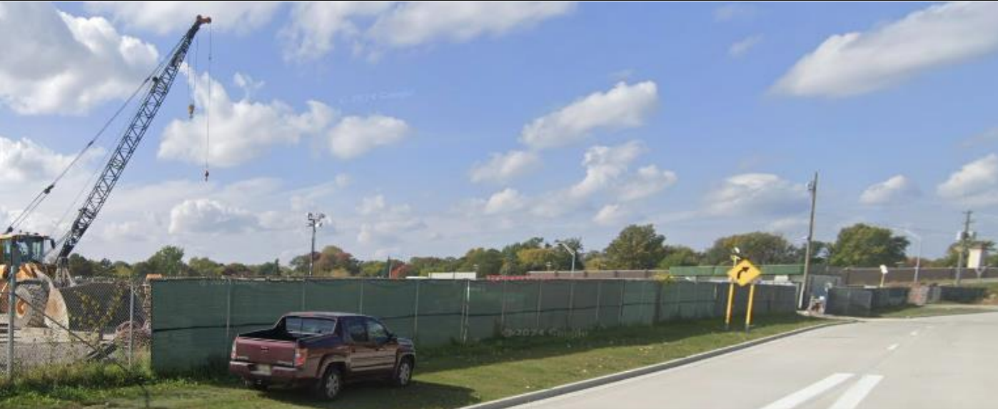
Example 1: Site Perimeter Shielded Fence
