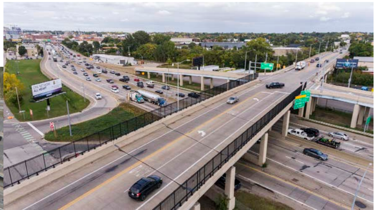
Martin Luther King Jr. Street (Franklin Street) bridge is outdated and in need of repairs
