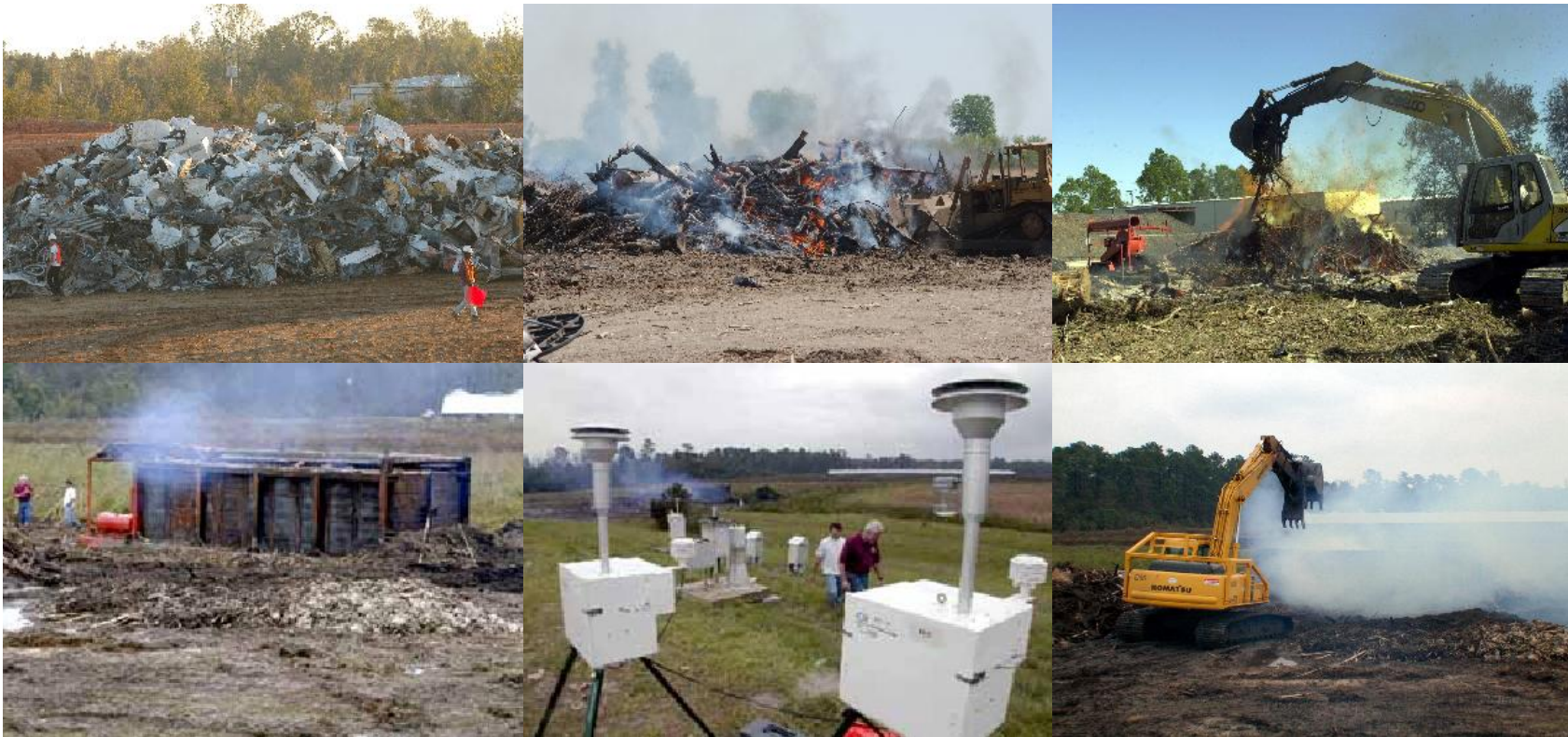
Clockwise, from upper left: Debris pile prior to volume reduction; open air, controlled burn pile; air curtain burner; portable incinerator; air monitoring equipment at burn site; open air, controlled burn pit.
