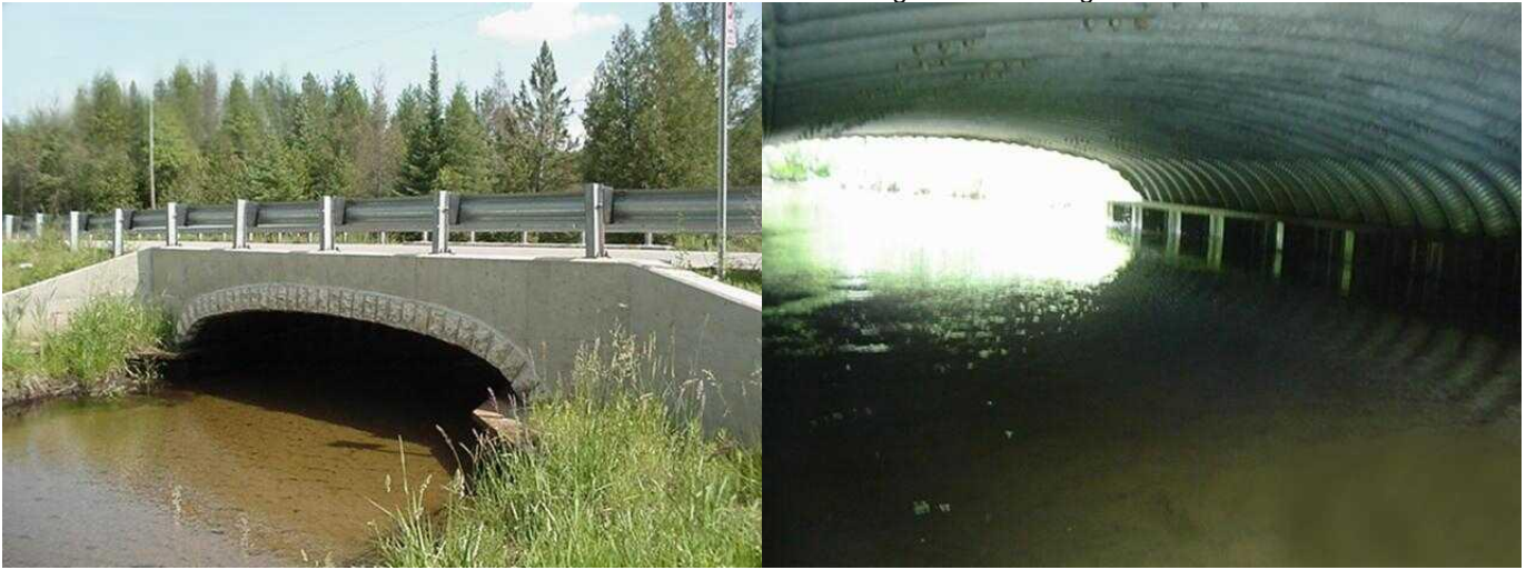
Photos L-R show the new 22-foot box culvert which replaced an inadequate twin culvert system. Concrete headwalls were also installed and stream bank stabilization measures, such as rip-rap, were taken.
