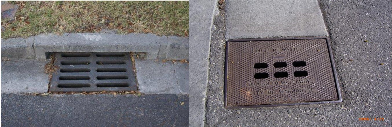
Photos L-R: Pre-construction – non-restricted catch basin cover. Post Construction – example of one of the 2,300 restricted catch basin covers installed throughout the City of Wyandotte.
