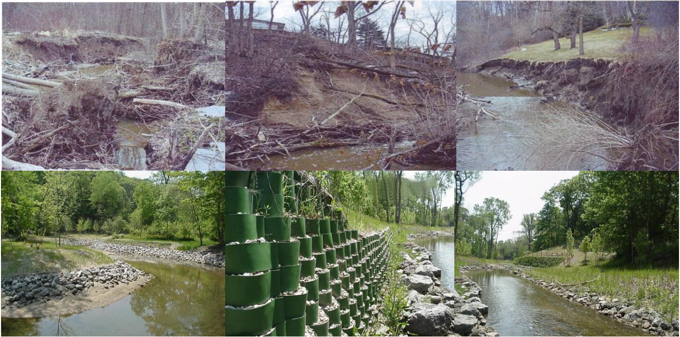
Top Row L-R: Prior to the project, major sections of the Franklin Branch suffered severe erosion and deterioration which threatened homes, businesses and infrastructure. Bottom Row L-R: The new stream bank stabilization measures will help prevent bank erosion, improve water quality, and protect nearby homes, businesses and infrastructure.
