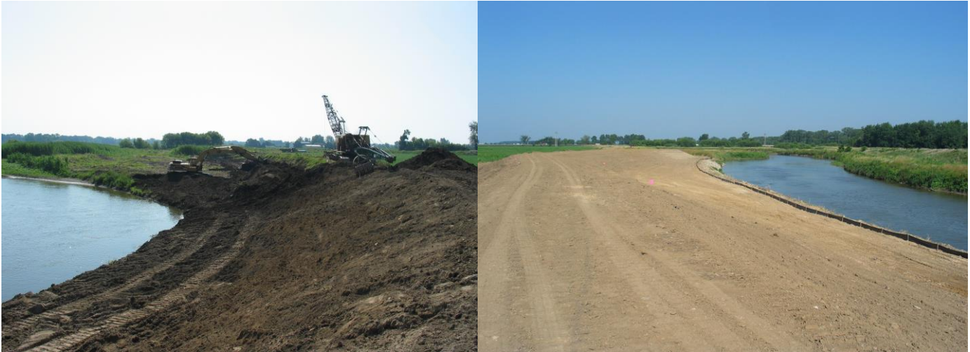
Photos L-R: A section of the dike under construction in Saginaw County; a reconstructed section of the dike, before final grading and reseeding. The new dike is constructed to modern standards with a wider course, 1:4 slope setbacks, and a series of detention areas and flood spillways to accommodate excessive flow.
