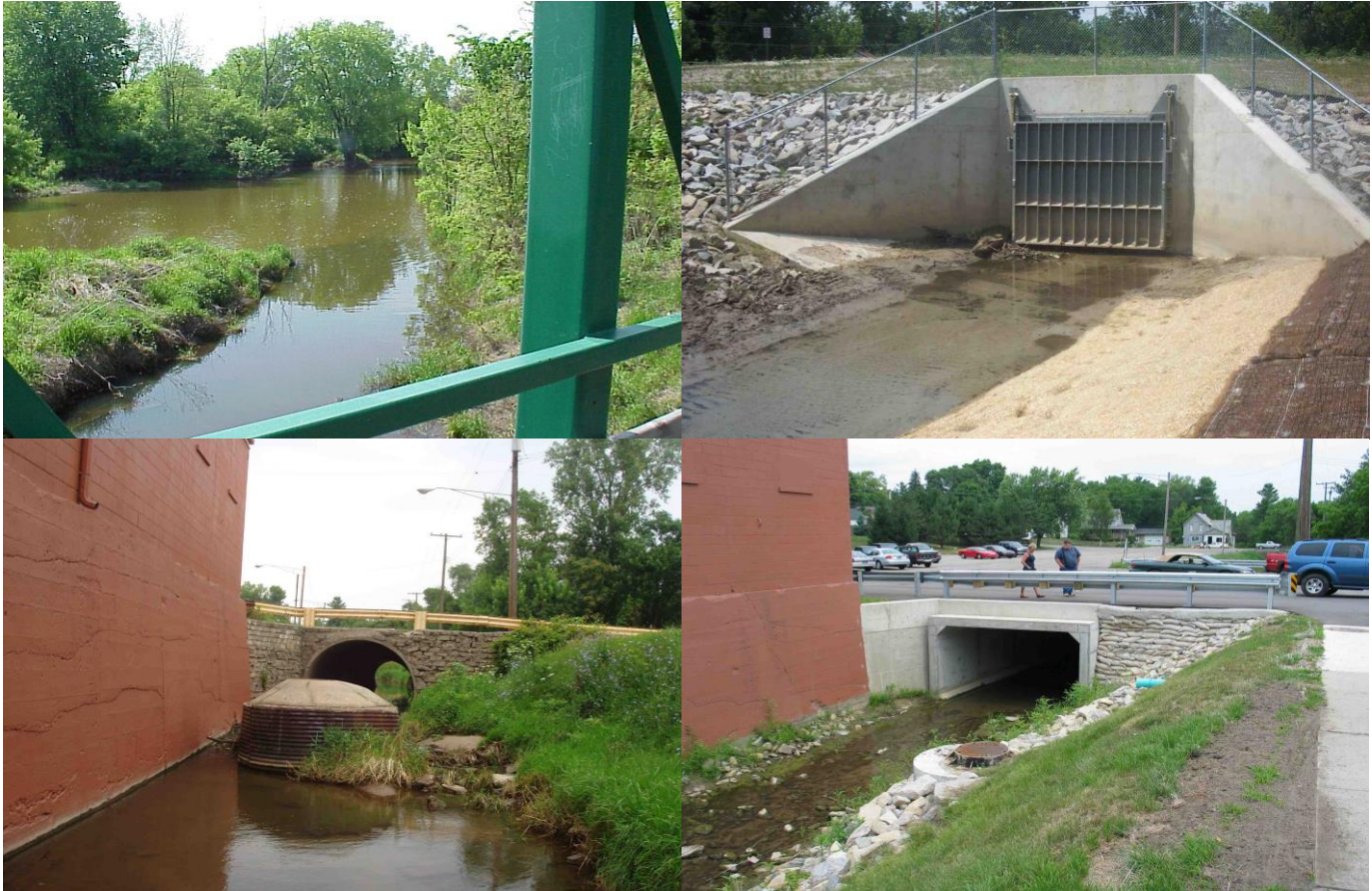
Top Row L-R: Pre-construction – Moore Drain outlet to Cass River with no outlet structure; Post-construction – Moore Drain outlet to Cass River (new) with backflow flap gate; Bottom Row L-R: Pre-construction – Moore Drain downtown parking lot culvert (inadequate); Post-construction – Moore Drain downtown parking lot culvert (improved).
