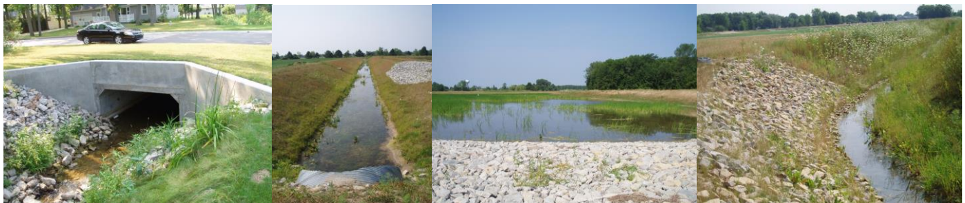
Photos L-R: View of new culvert with wing walls; improved drain channel with rip-rap overflow; view of detention pond; inlet channel with erosion control.
