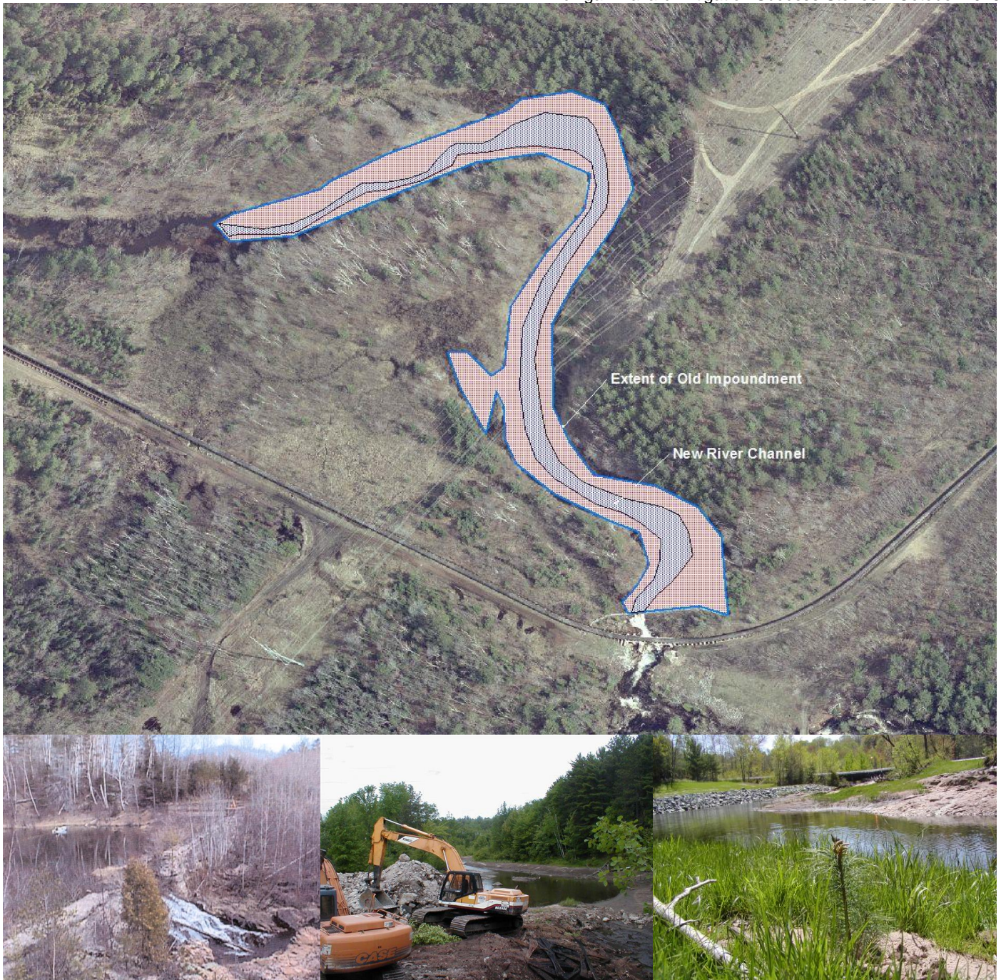
Top Row: Aerial photo depicts the old impoundment and new river channel. Bottom Row L-R: Collinsville Dam before removal; excavators removing the dam; re-vegetation and rip-rap along the river after dam removal.
