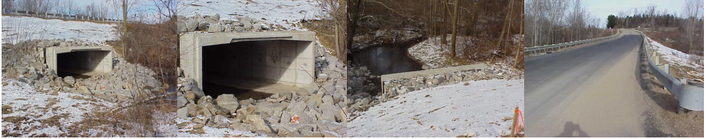
Photos L-R show the new box culvert, stream bank stabilization measures, and roadway enhancements which are designed to improve drainage and better protect the roadway infrastructure.
