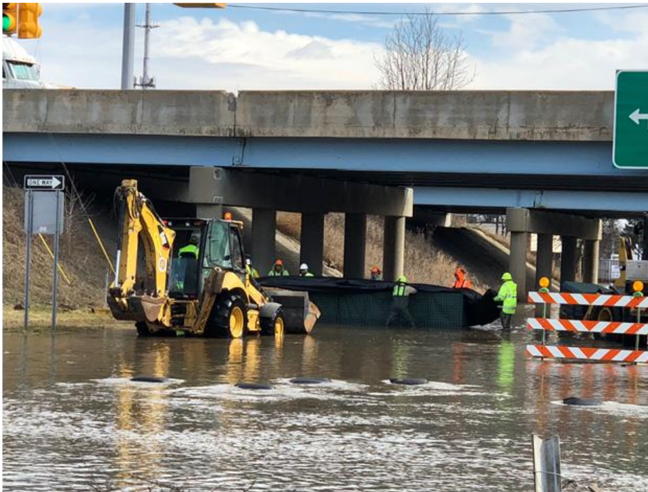
Photo: Workers in Lansing build a temporary flood barrier at the Kalamazoo Street underpass of US-127.
