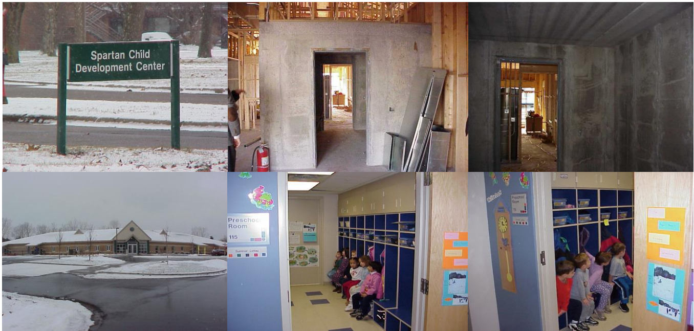
Top Row L-R: Storm rooms during construction. Bottom Row L-R: Storm rooms as they appear today in their completed form (disguised as coat rooms).
