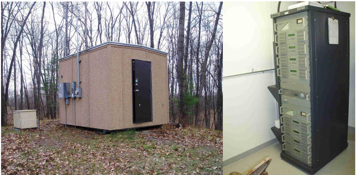
Photos L-R: Transmitter equipment building with back-up generator; transmission equipment inside transmitter equipment building.
