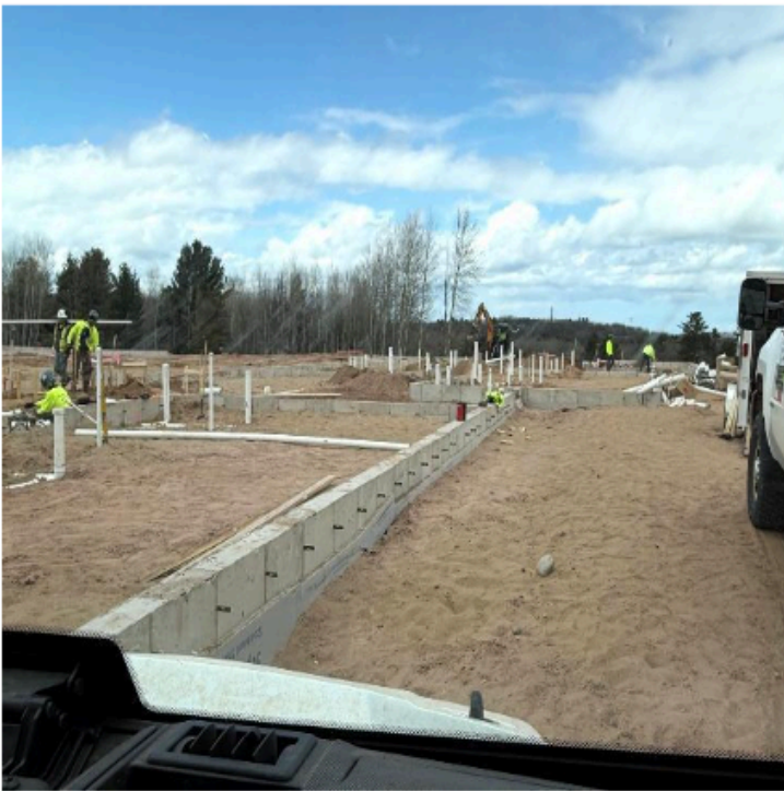
Shallow Underground Plumbing
