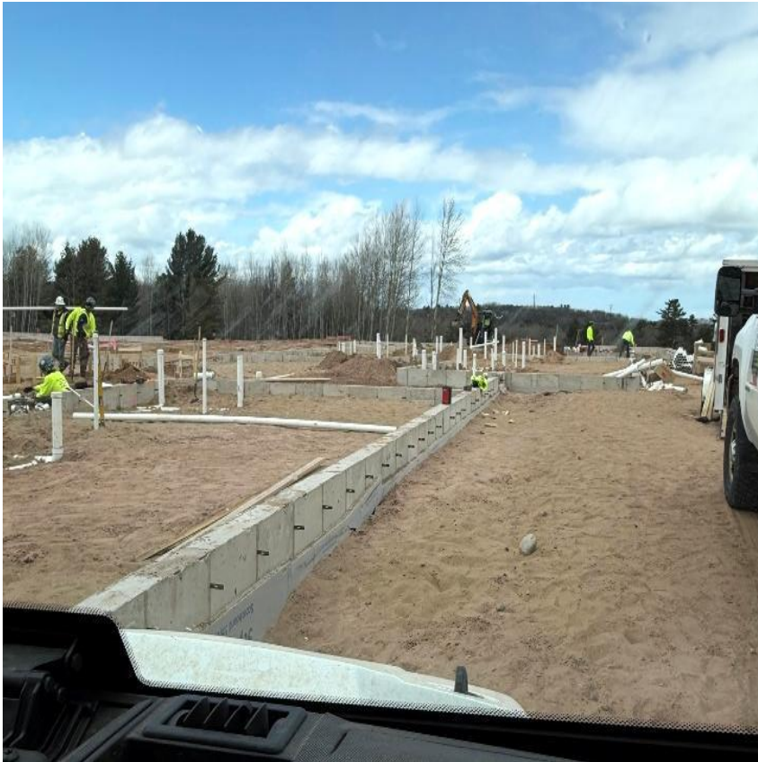
Shallow Underground Plumbing
